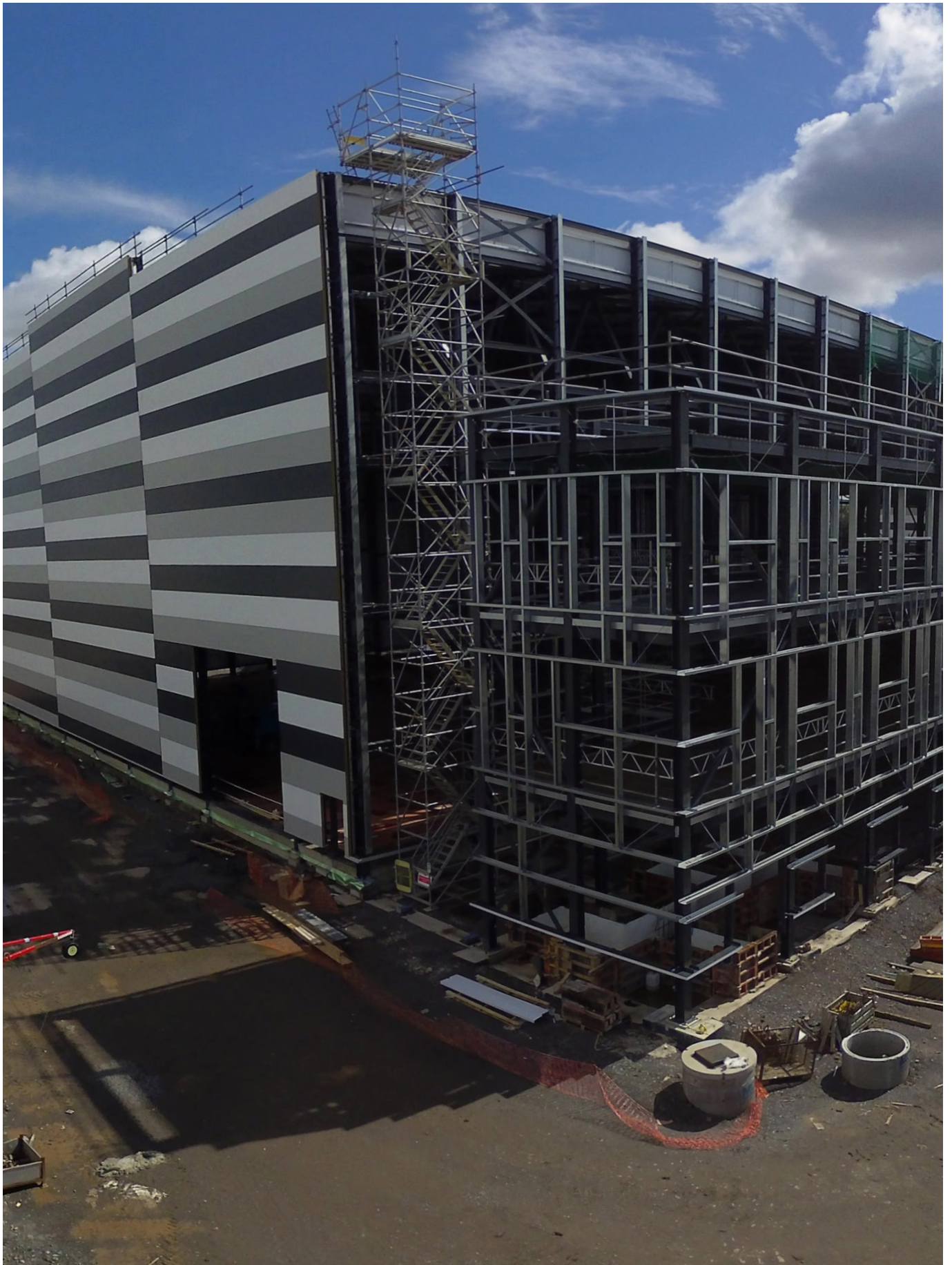
FIG 1 STUDIO ULSTER CURRENTLY UNDER CONSTRUCTION AT BELFAST HARBOUR STUDIOS, BELFAST, N. IRELAND JUNE
